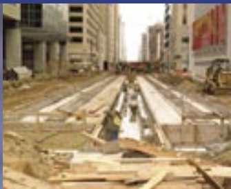
City of Houston Main Street Square Fountain & METRO Light Rail Line. Civil Contractor: Texas Sterling Construction, L.P. Photo: Metropolitan Transit Authority.
